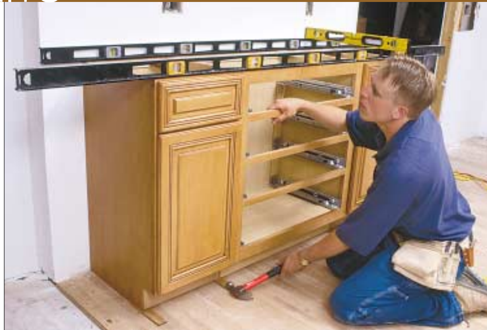
Check for level along the front face and from front to back, especially when working on a section that meets another unit in a corner.
