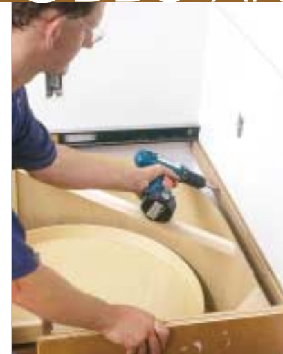
Corner cabinets with curved backs are made for fitting through 36-in. doorways. However, unlike corner units made with mitered backs, they need extra ledger boards attached in the corner to support the countertop.
