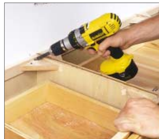
Attach base units to the wall with 2-1/2-in. self-tapping flathead wood screws, driving through the nailing strip and into studs. In this case, the stud fell behind a corner block.
